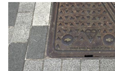
Access cover integrated into paving with minimal infill
