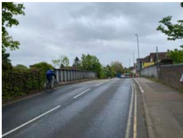
Figure 89. Missing footway on the bridge above the railway lines
