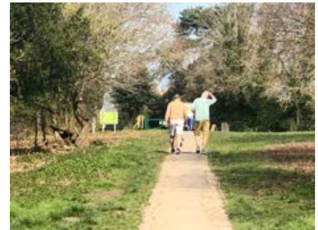
Figure 95. Narrow footpath with some defects through Farnham Park limits the accessibility to all.
