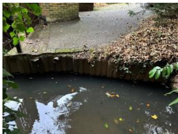
Photo 7 :Example of outlet into the stream from private property at Linersh Road.
