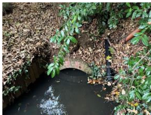
Photo 8:Image of culvert at Linersh Road showing multiple pipes entering the stream. It is unclear which relate to private discharge or Highways.
